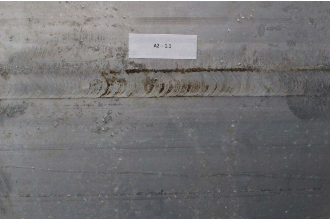
Figure 5: Corrosive Staining at Weld A2
