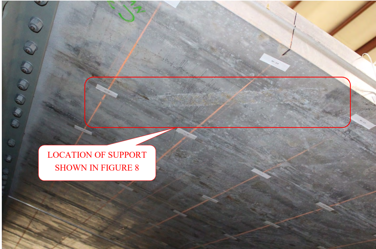
Figure 7: Corrosive Staining at Generation I Panel
