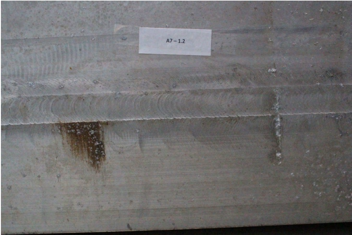
Figure 6: Corrosive Staining at Weld A7
