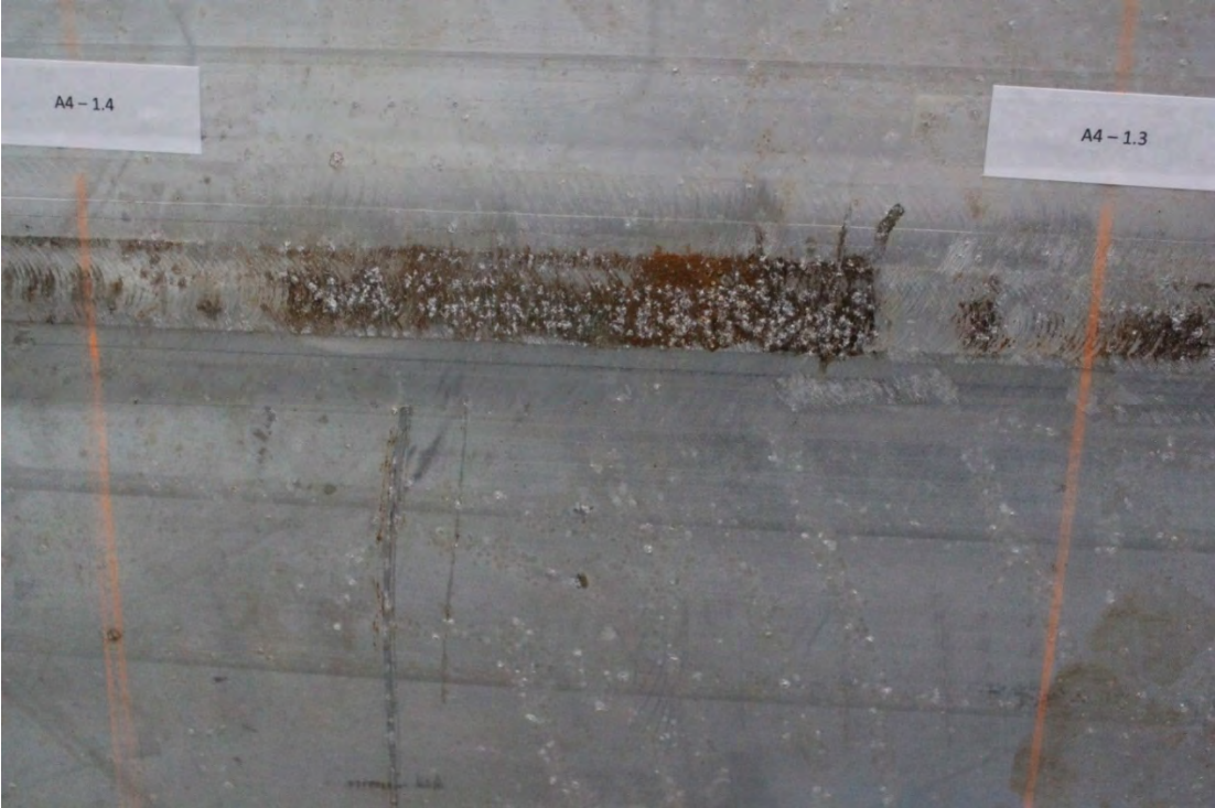
Figure 4: Corrosive Staining at Weld A4
